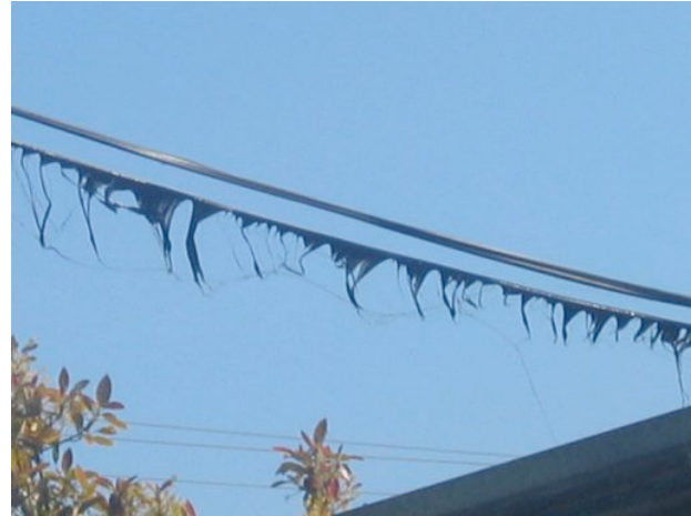
Ground Bonding gone wrong
